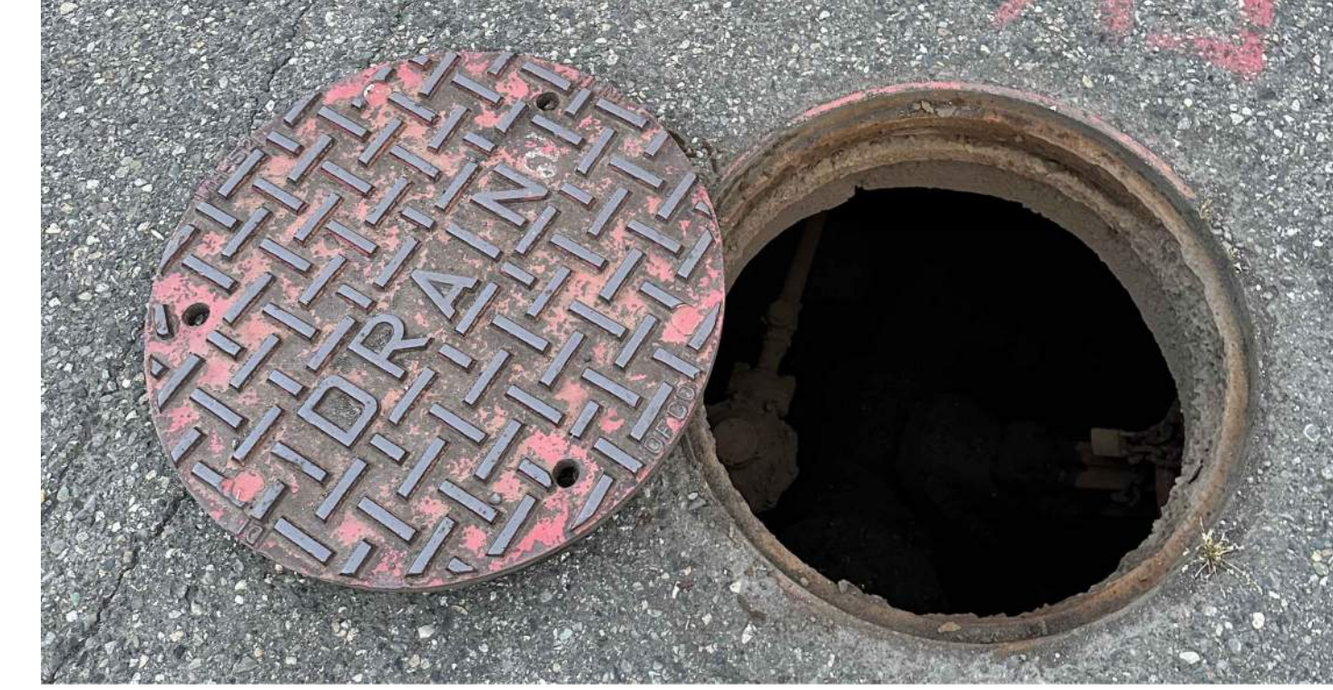
2 - PHOTO - EX WATER METER VAULT LID
